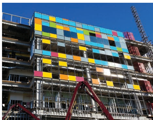
The new 89,000-square-foot Center for Advanced Outpatient Care will be completed in Fall 2017.
